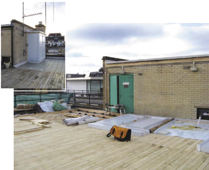
Terrace decking being laid on protective geotextile and rubber pads. Larch bearers support sweet chestnut decking. Inset: new porch for easier access by staff.
