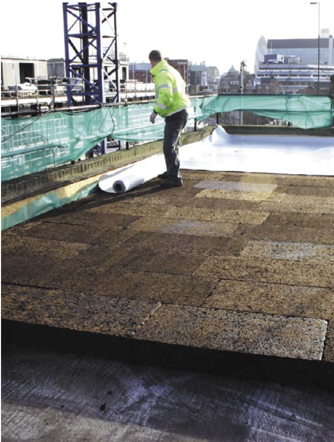
The cork board being laid over the existing asphalt roof with the new waterproof membrane being laid over it.
