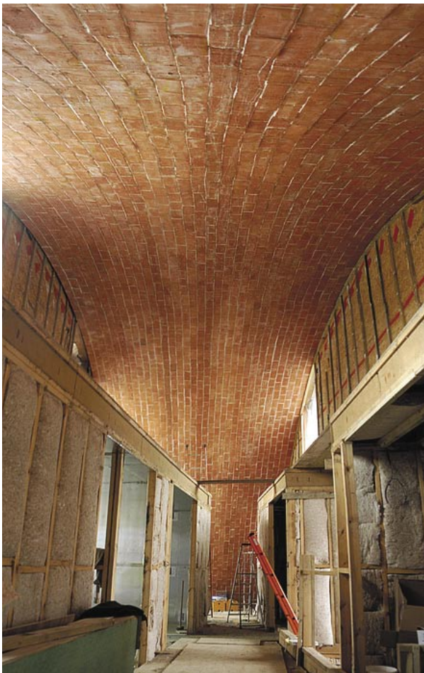
Right: Crossways, Staplehurst where the architect, Richard Hawkes, has designed himself a new house based on an arch enclosing a cluster of cubical shapes. The method of constructing the arch was uncertain, until Andrew Bassant, of Ecolibrium Solutions, recommended timbrel vaulting. Richard Hawkes became enthused by the idea and found a local pottery, Babylon, to fabricate them using local clay usually used for Kent peg tiles.
