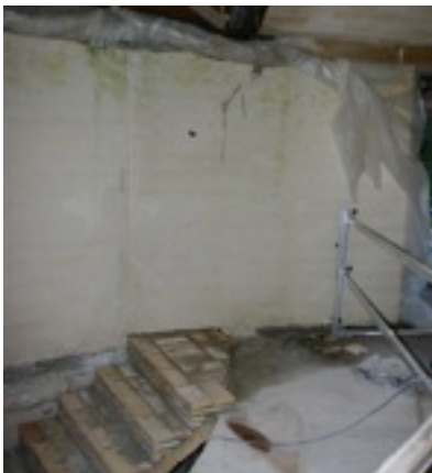
8. Plaster protection rolled up to allow drying. Note staining
