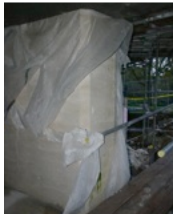
9. Light plastic protection damaged by wind
