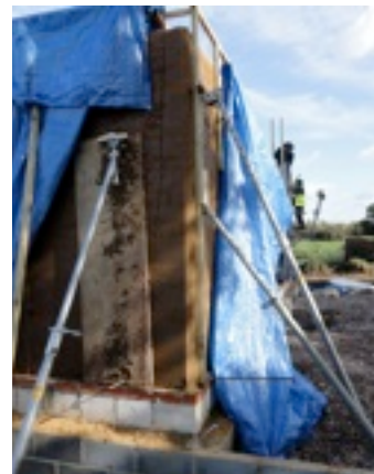
10. Wall damaged by over-zealous propping
