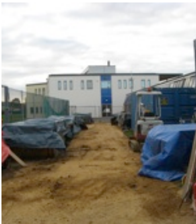
3. Earth stored in covered skips - high risk of covers letting in water and saturating material
