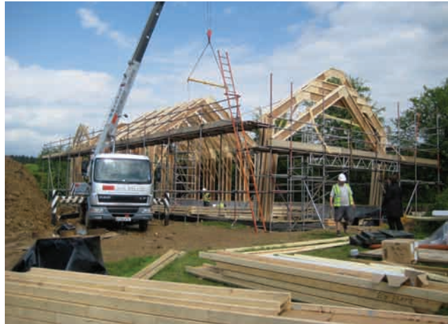
The portal frame installation went smoothly and the open interior design made it simpler for the contractors to achieve airtightness.
