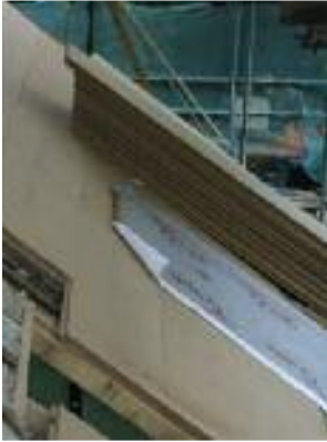
Left: Insulation boards applied over rafters, with wool between, with a Tyvek membrane, counter battens and battens
